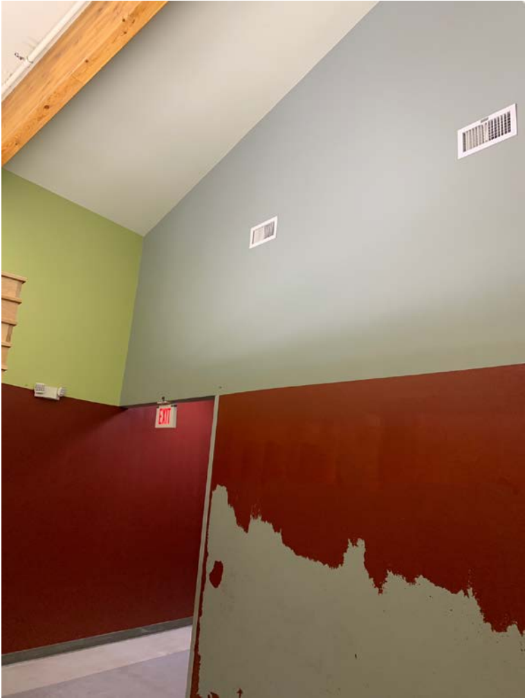
Peeling Loose Paint
