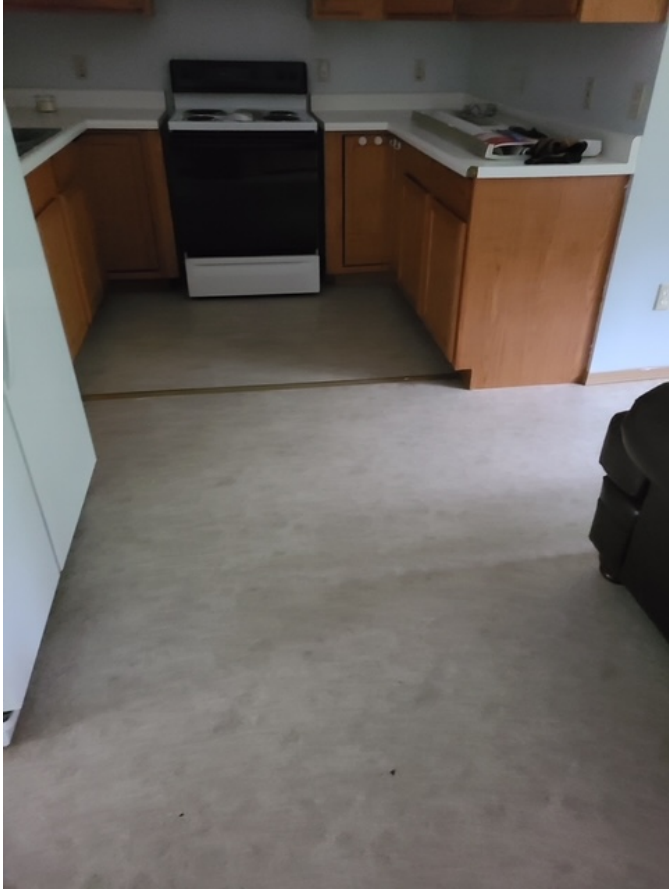
Previous Damaged Flooring
